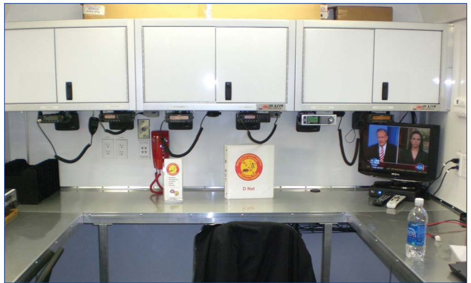
The communications room in the mobile command center was designed and had its equipment installed by a local amateur radio group.
